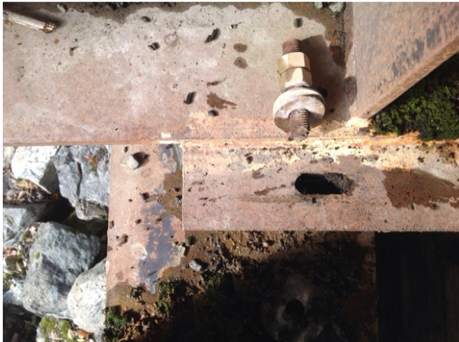
right bank upstream bearing bolts (both) sheared off
